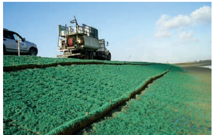
OVER 34 ACRES of various hydroseed mixes were applied to the slopes at Bolsa Chica.
