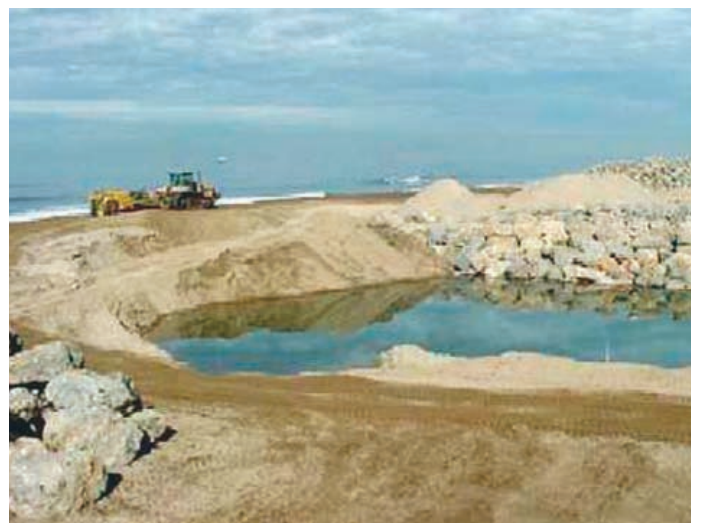
PRECISION OPERATION – Construction work such as grading, placing of Rip Rap and landscaping required precision operators to work next to the ocean and Pacific Coast Highway.
