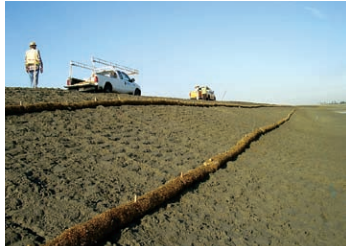
EROSION CONTROL – Over 35 miles of straw wattles were installed per specifications, and within the project's demanding schedule!
